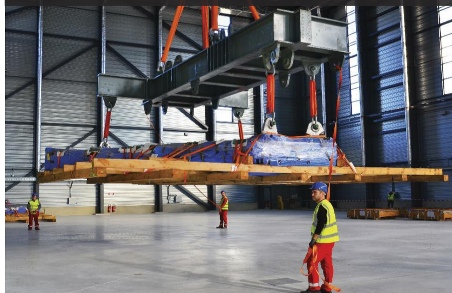
Six of the components that reached ITER in December weighed 50 tonnes each. Assembled with six auxiliary segments and welded, they will form Tier 1 of the cryostat base, the heaviest single “piece” of the ITER machine (1,250 tonnes).
